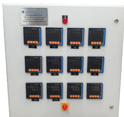
Plant Process Indication with SCADA/PLC Interface
